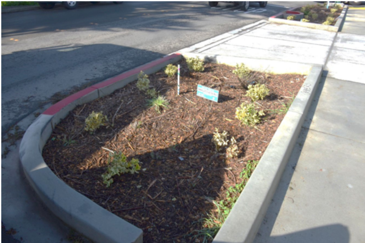
Newly installed green infrastructure along Palmetto Boulevard.
